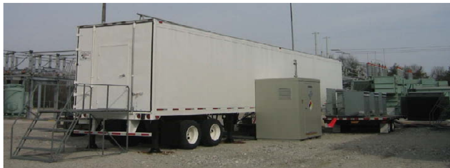
AES 1 MW substation energy storage system
